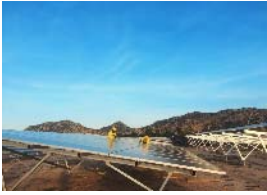
Hanh Nguyen, taken while working on the largest solar farm in Vietnam
