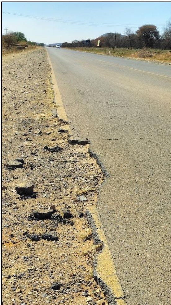
Road edge breakaway on D114 opposite site access road in need of repair (damage due to large vehicles turning right from gravel site access road and / or through traffic passing vehicles turning right into gravel site access road).
