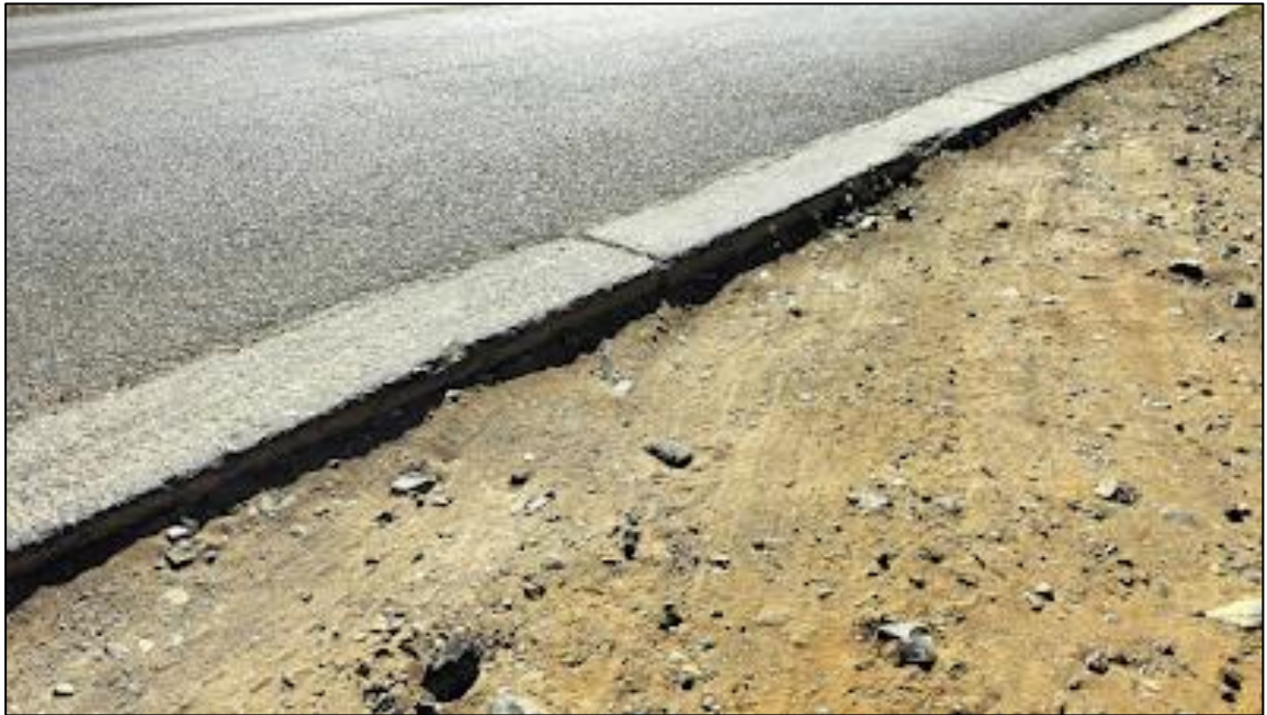
Concrete edge beam drop-off close to road edge poses a traffic danger to motorists
