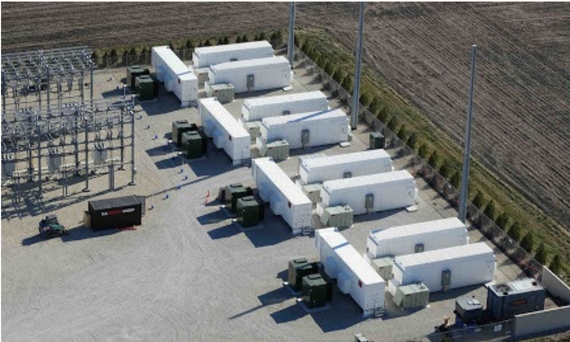
FIGURE 8-2 A STOCK IMAGE OF A SIMILAR DEVELOPMENT WITH AN ON-SITE SUBSTATION AND BESS
