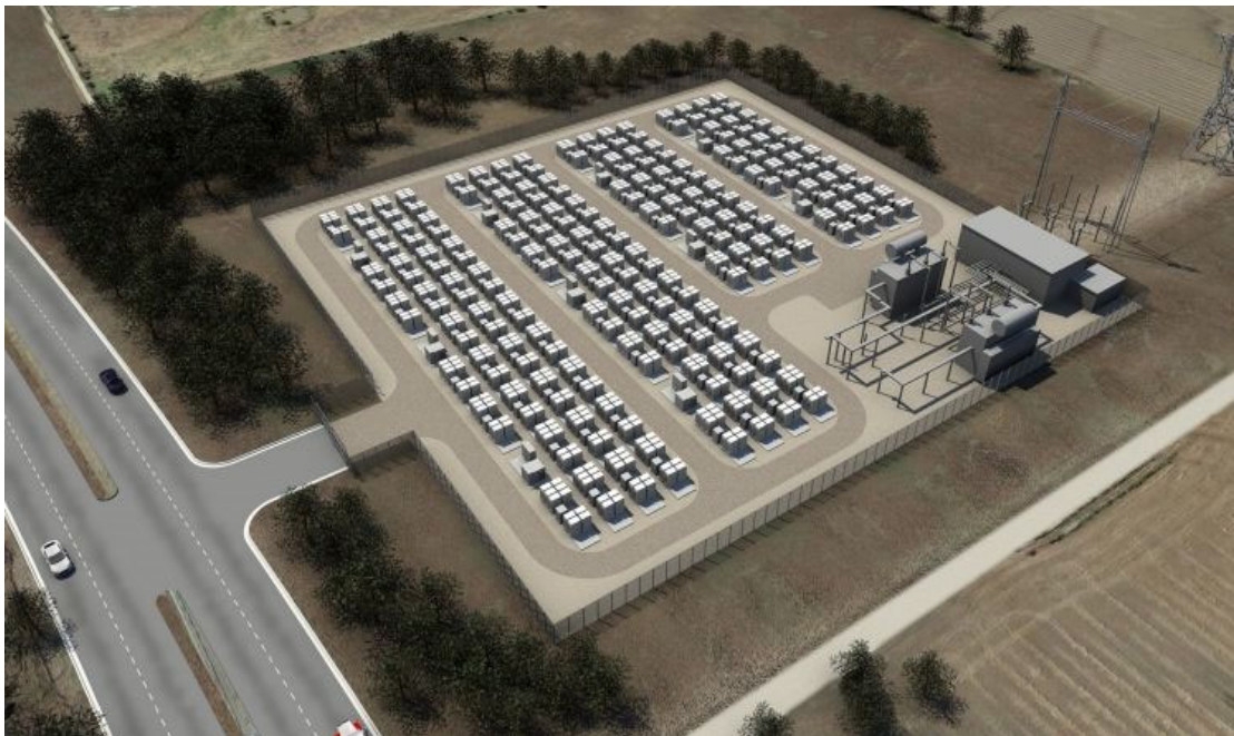
FIGURE 7-5 SOLARCITY'S TESLA BATTERY STORAGE FACILITY, HAWAII
