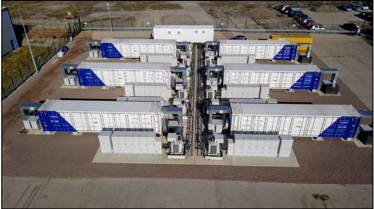
Photograph 1.2: Example of BESS located in storage containers
