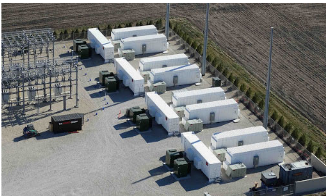
FIGURE 7-7 A STOCK IMAGE OF A SIMILAR DEVELOPMENT WITH AN ON-SITE SUBSTATION AND BESS
