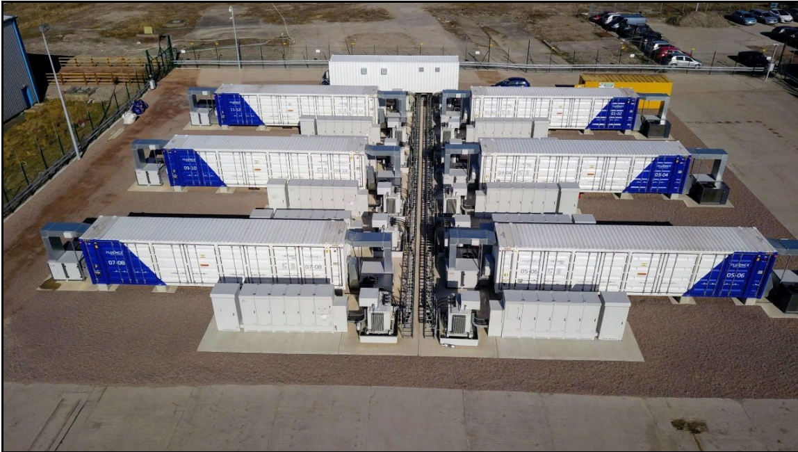
Photograph 1.2: Example of BESS located in storage containers
