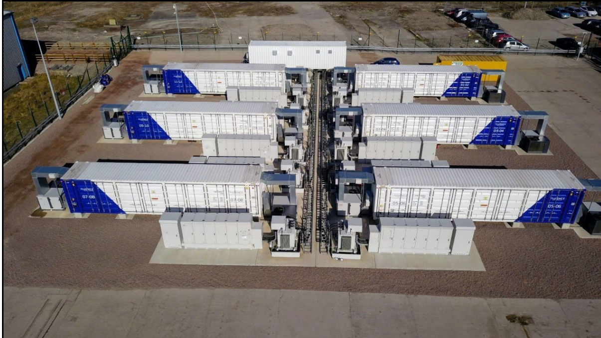
Photograph 1.2: Example of BESS located in storage containers
